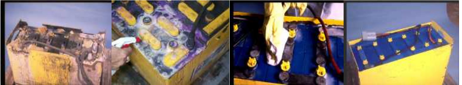
Fig.1 An example of a poorly maintained battery. This battery will require more charge time and, as a result, less work time.
